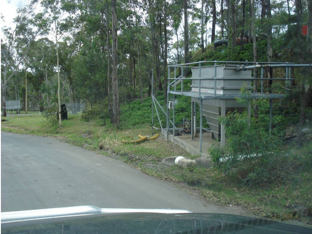
Plate 23 – Oil water separator – water from the facility is discharged via open drain to the main water dam below the pit top area (see photo below)
