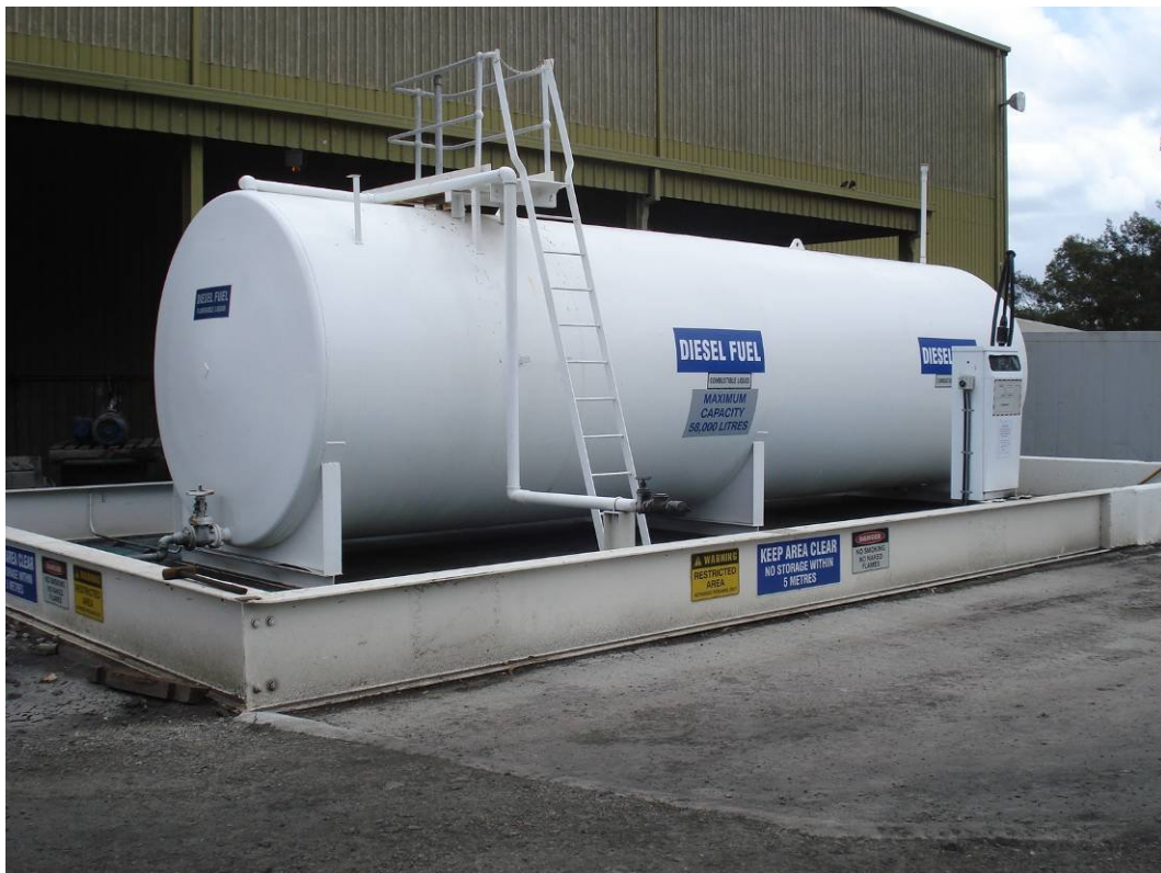
Plate 20 – Bulk Diesel storage tank.
