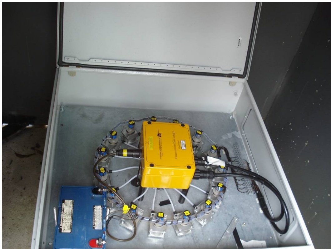
Plate 4 – Extensometer Data Logger over the existing Longwall Panel
