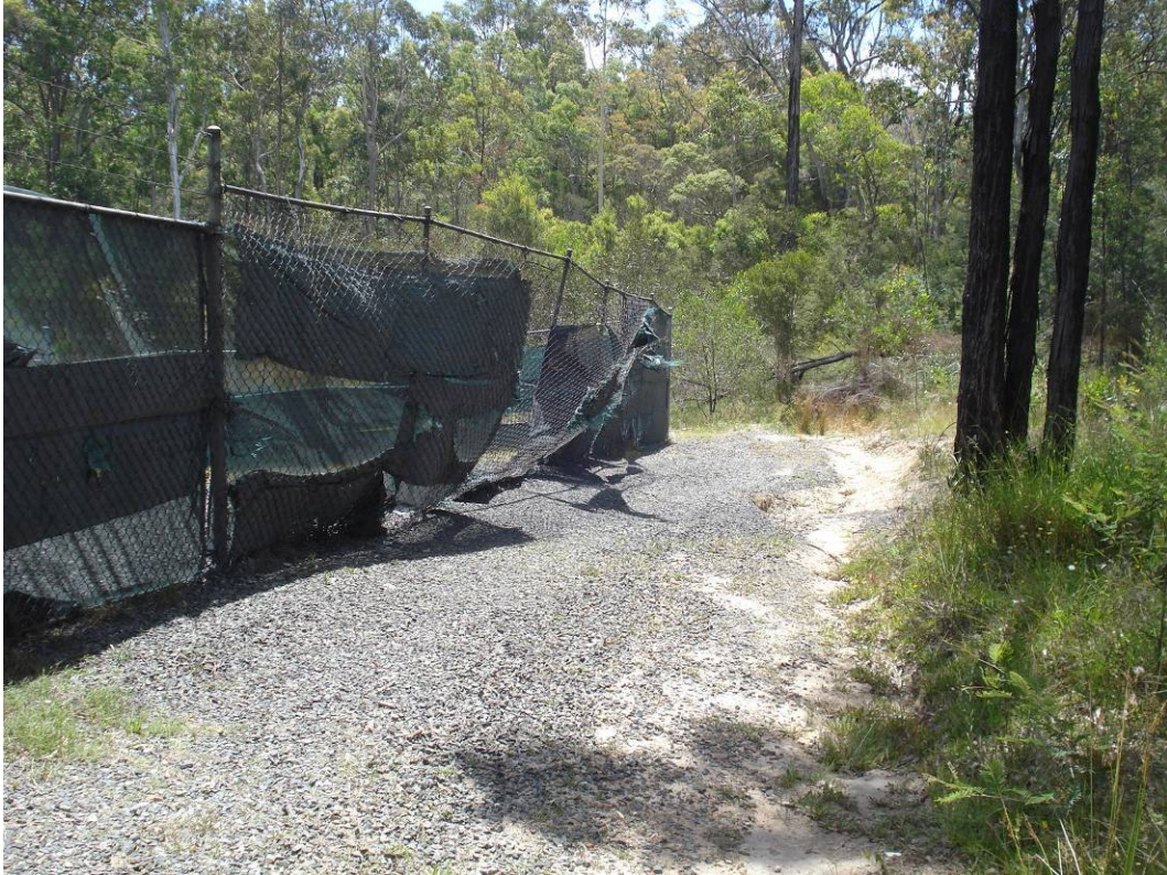
Plate 11 – Shade cloth on the security fence that has been installed to contain fines blown from the vent shafts. This was considered ineffective
