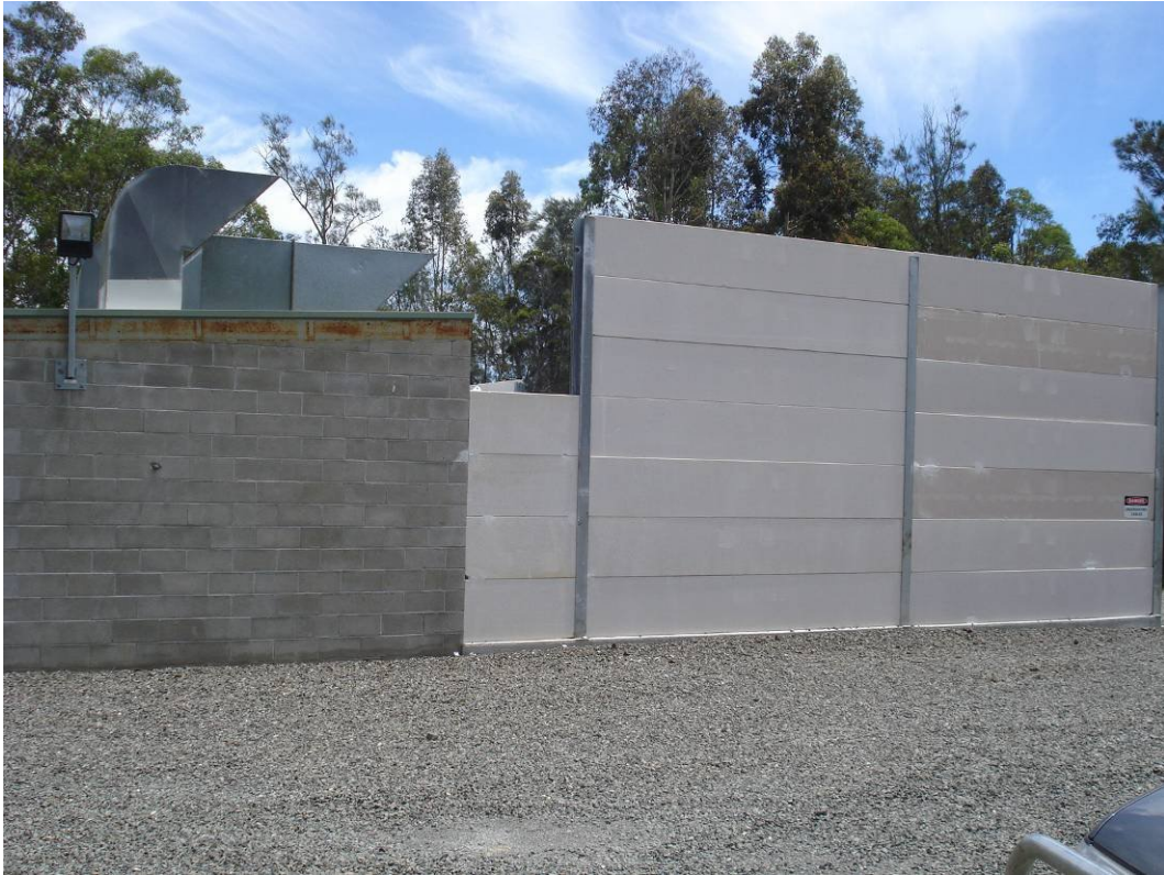
Plate 7 – Vent fans with noise mitigation bunding
