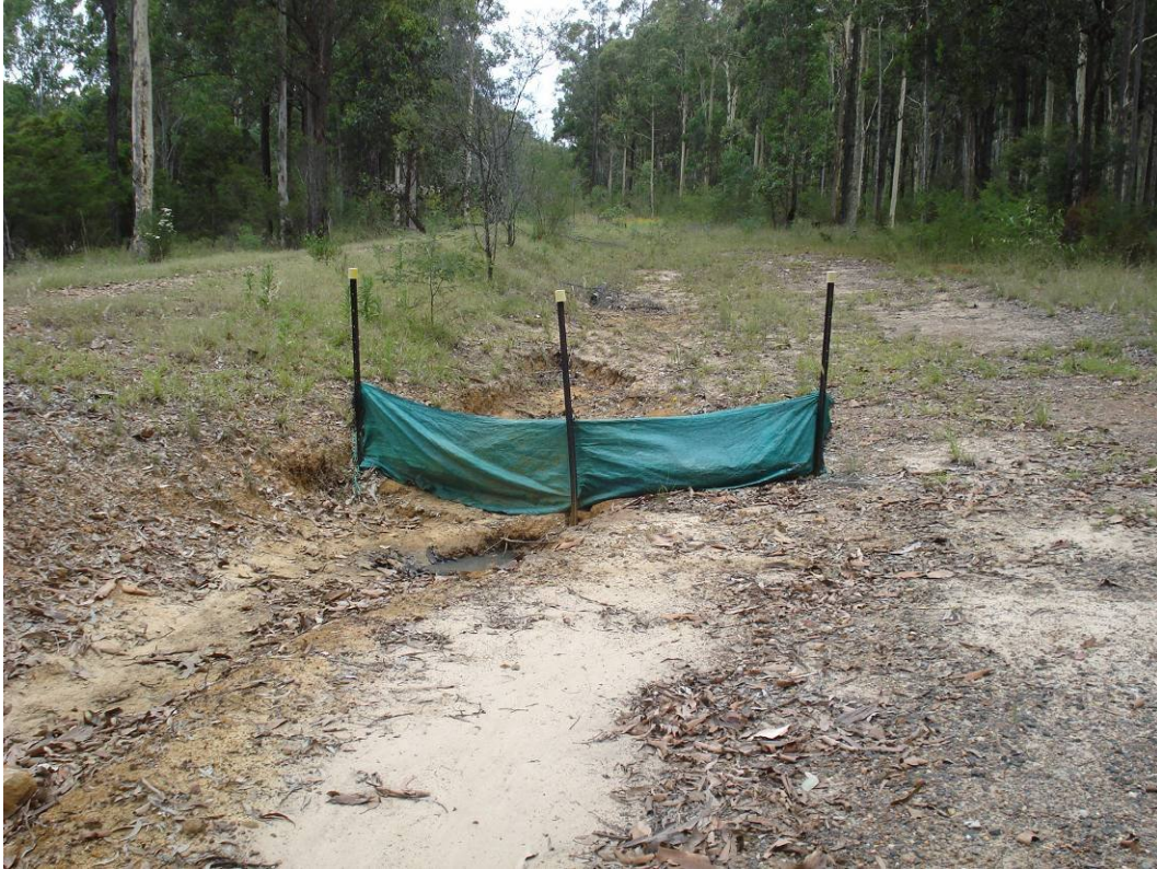
Plate 25 – Silt fence in a clean water diversion drain around the dam. The construction of the silt fence was considered poor and as a result it was considered ineffective
