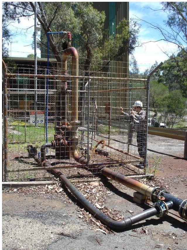
Plate 12 – Part of the underground water management system returning water from the underground to the Coal Preparation Plant.
