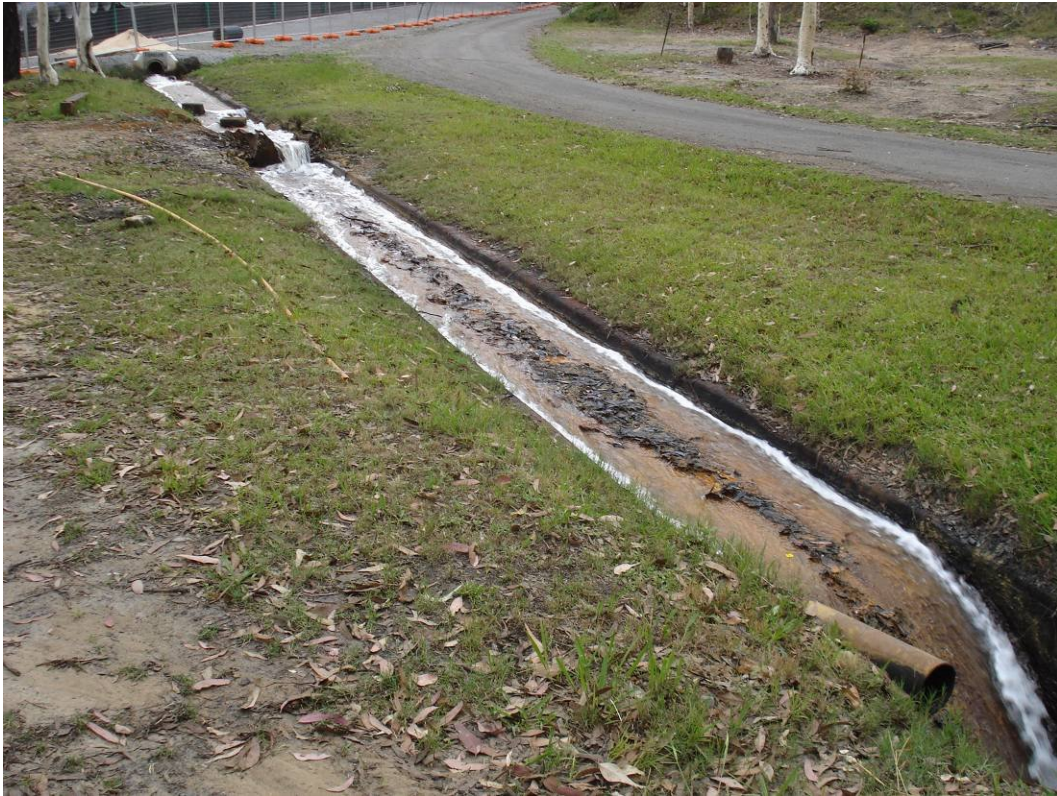
Plate 19 – Drain that transfer water from the underground to the Austar dam. Part of the underground water management system
