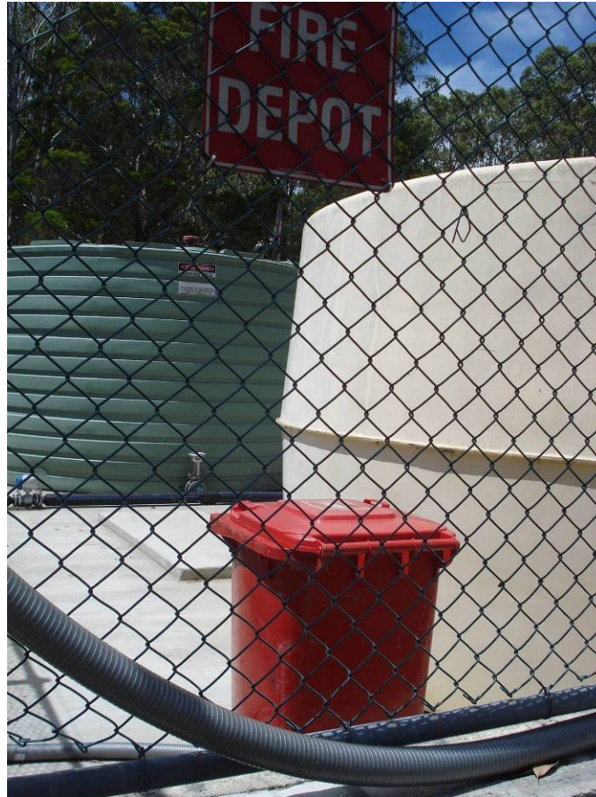
Plate 9 – Spill Kit within the bunded tank area
