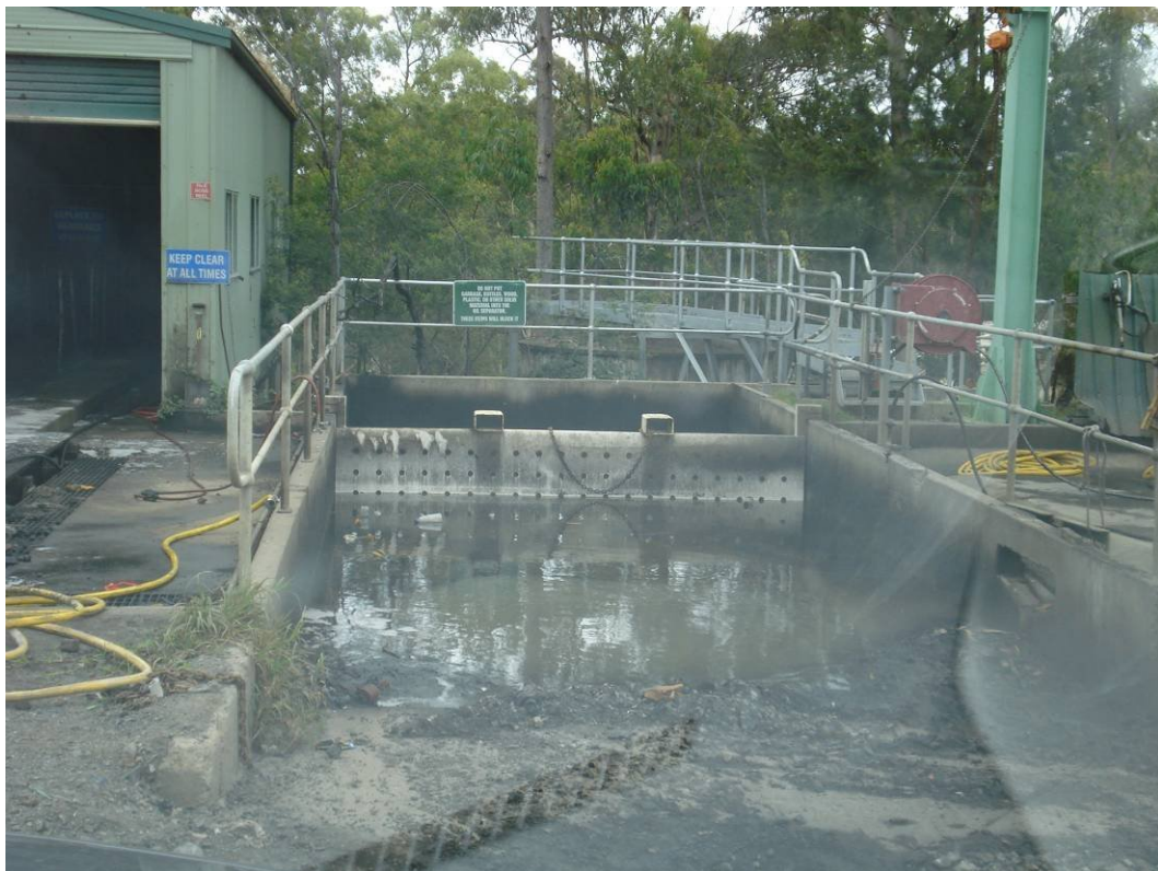
Plate 22 – Wash down pad and sediment sump. Water from this area passes through a triple interceptor before flowing onto an oil water separator.
