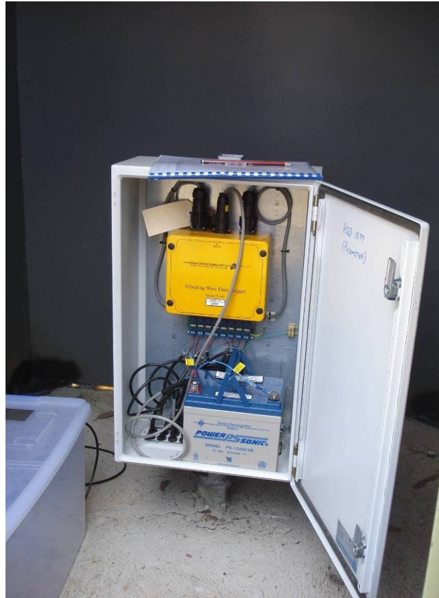
Plate 3 – Vibrating Wire Monitoring Data Logger over the existing Longwall Panel
