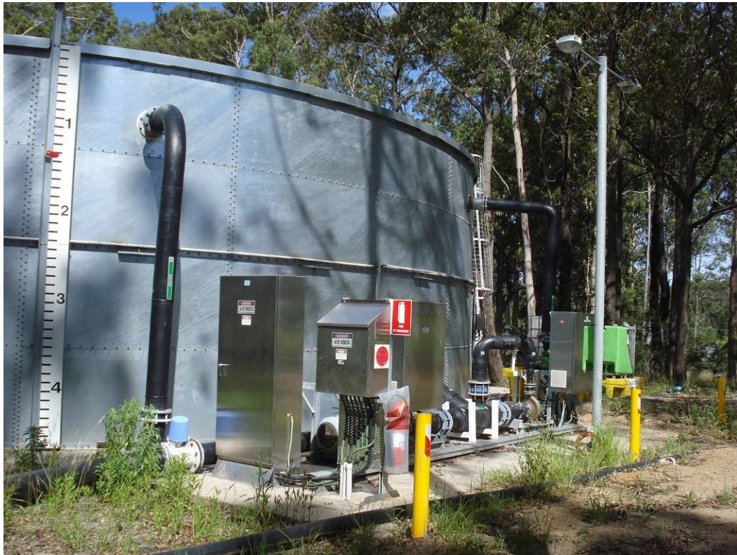
Plate 15 – Final storage tank and water treatment point prior to being discharged from the site at the licensed discharge point
