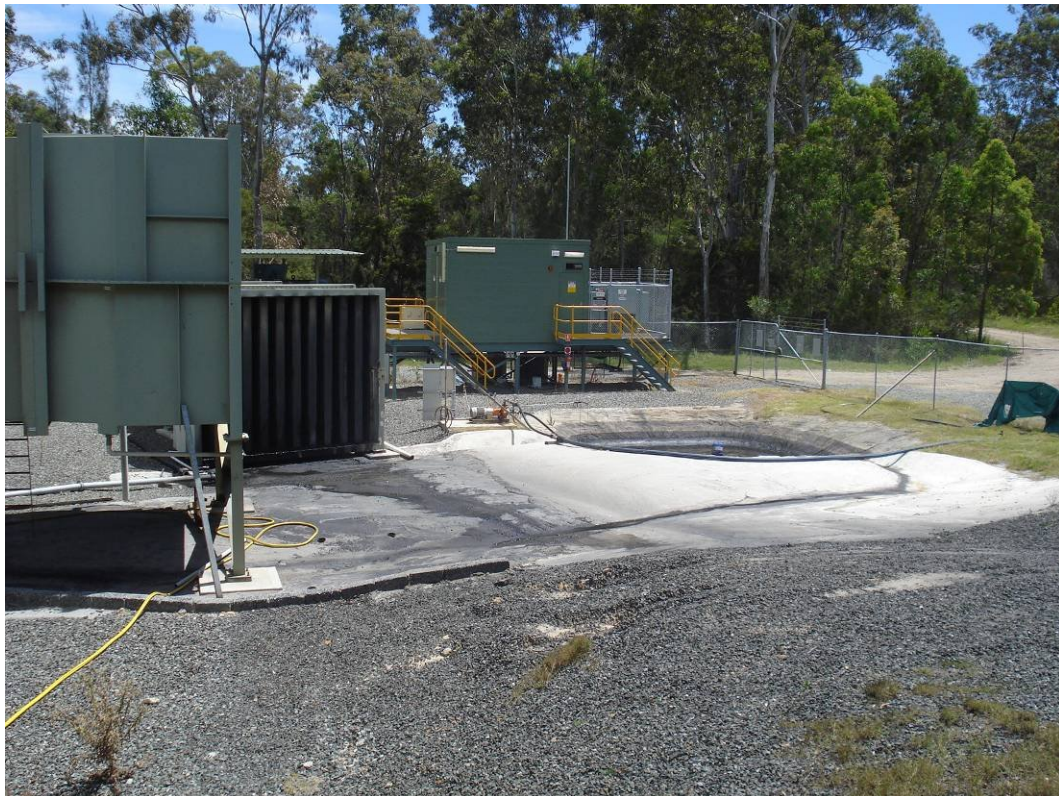
Plate 10 – Vent shaft with direction of shaft facing away from the neighbours. Note the sump installed to collect and retain condensation from the vent fan.
