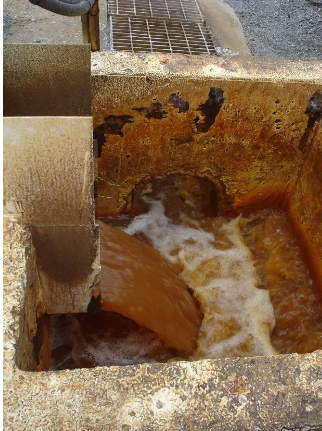
Plate 33 – Water being discharged to the settlement dam following treatment
