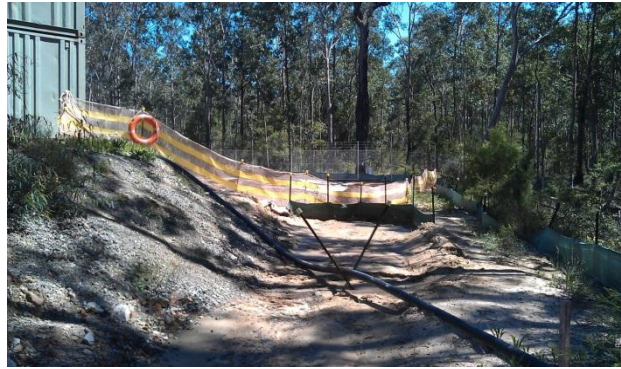
Figure 4.6B: Remove sediment fence from inlet to basin. It acts as a dam.
